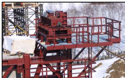
▲ Sliding bearing and lateral guides.
