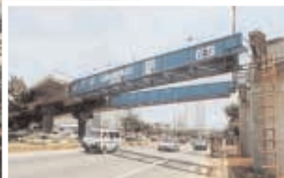
Overall bridge with casting yard in the background, and launching nose position before reaching the pier, spanning the main street of Sudirman
