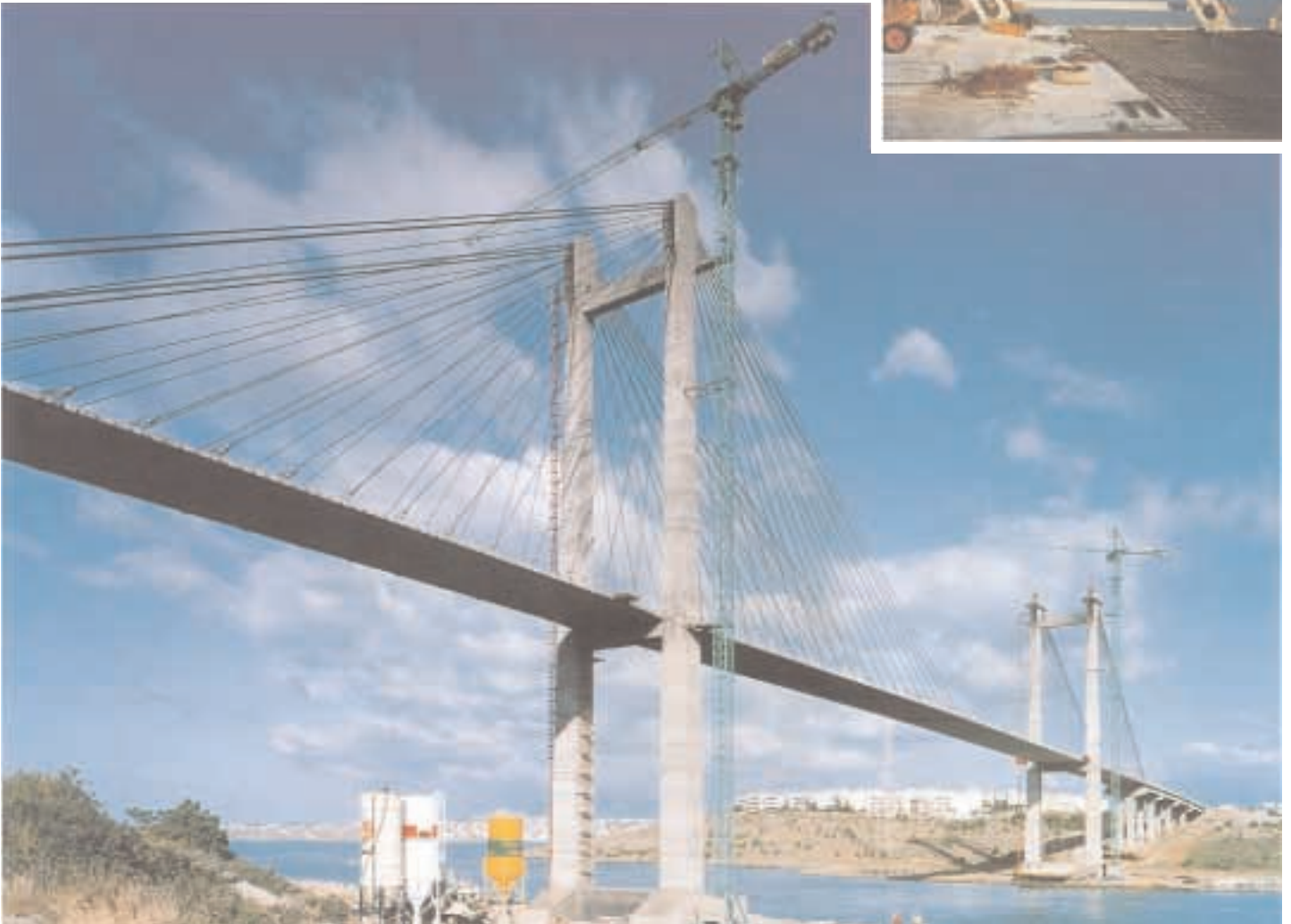
A view of the bridge following cable installation. Detail : The exposed deck anchorages
