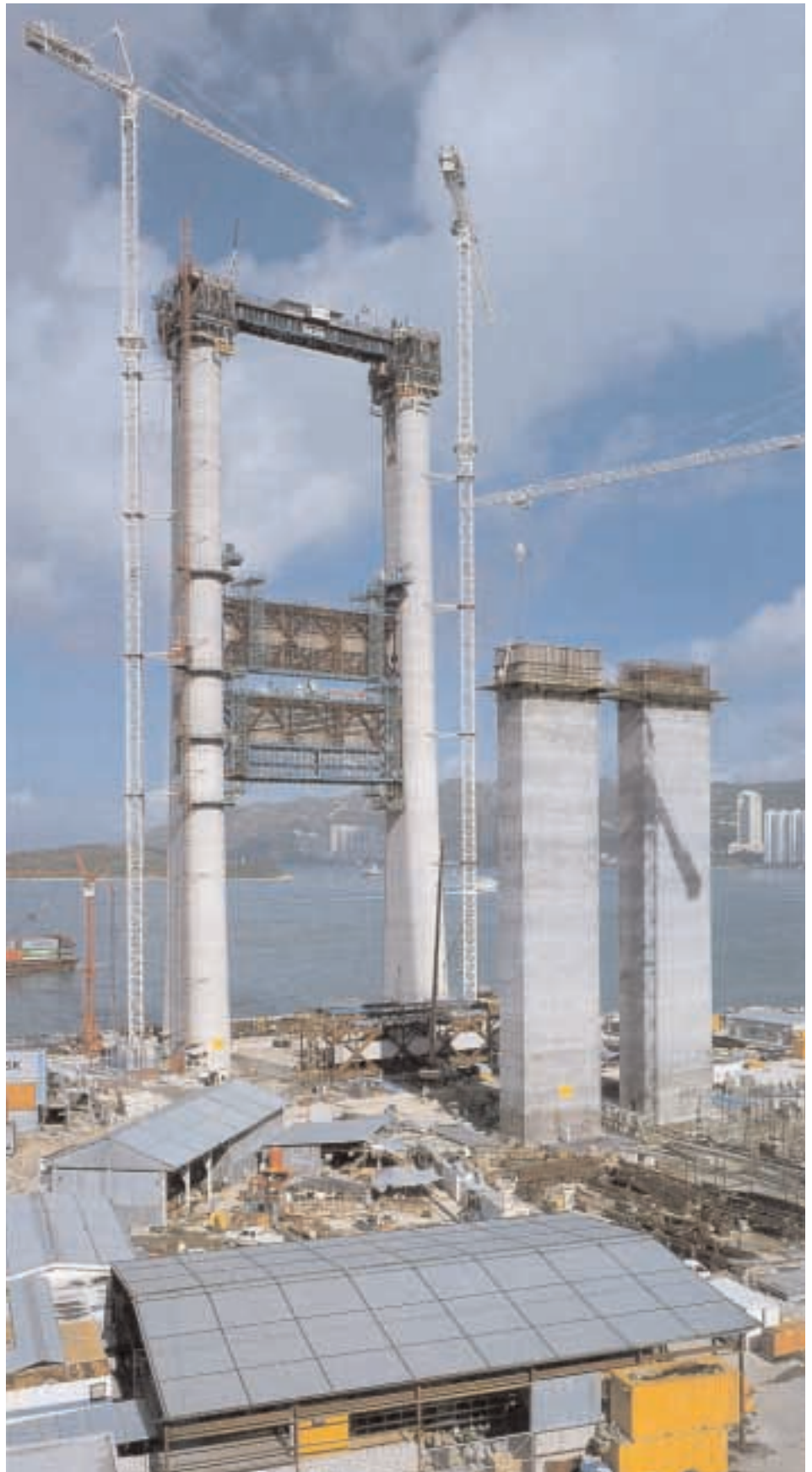
The fast growing Tsing Yi Tower at a height of 150 m with one of the piers in the foreground
