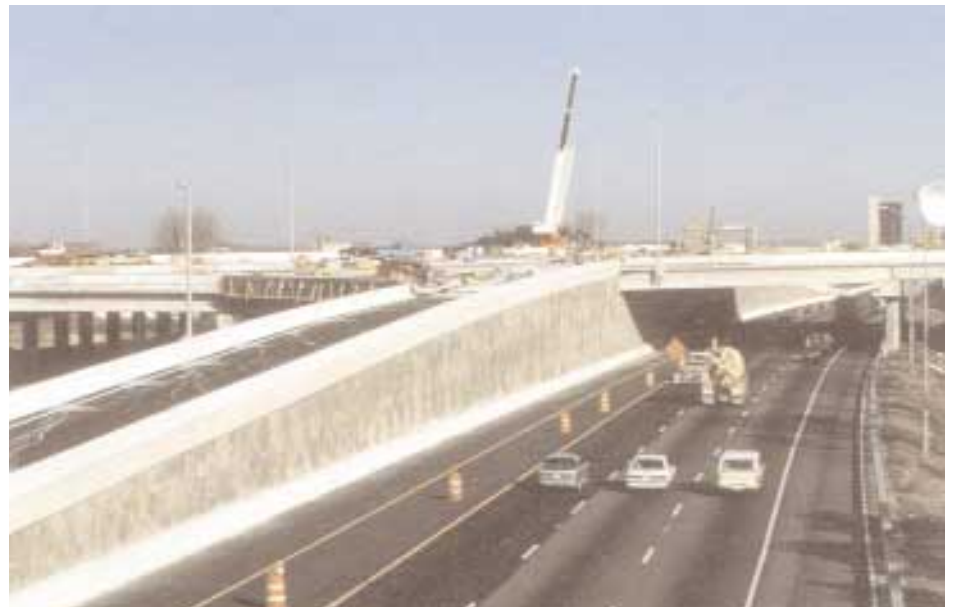
Retained Earth fractured fin panels support access ramps from Springfield Parkway on Interstate 95.
