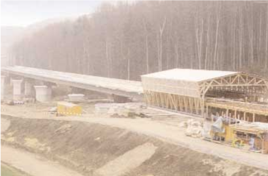
The incremental launching method offers improved quality because of shop like fabrication conditions, as well as economy.
