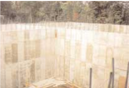
With suitable design, even multicell rectangular tanks can reap the advantages of post-tensioning.
