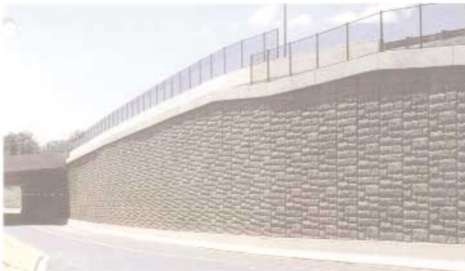
Retained Earth "Ashlar Stone" panels support access ramps for I-270 near Washington, D.C.
