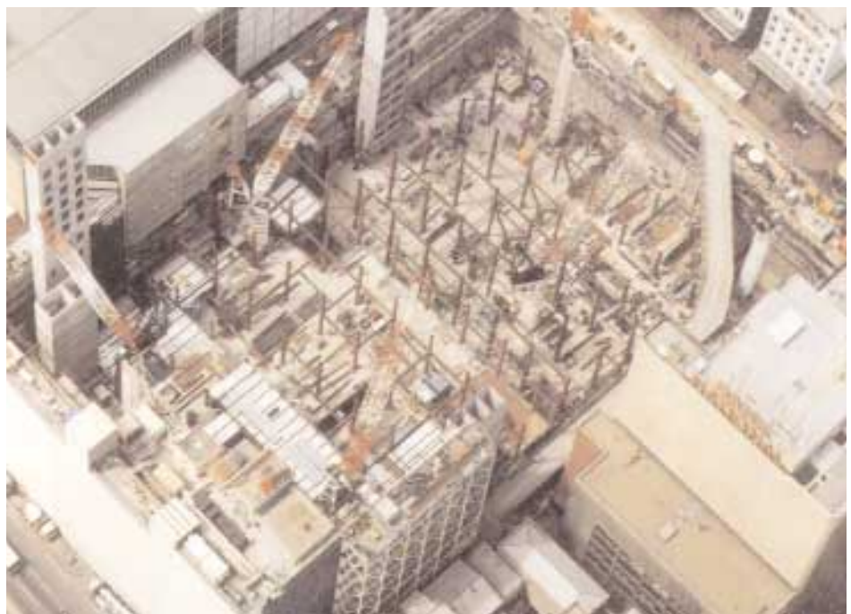
VSL alternative slab design successfully combined structural steel shear heads with the area's seismic reinforcement requirements.
