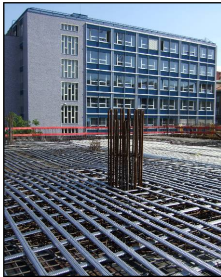
▲ PT tendons in the column area
