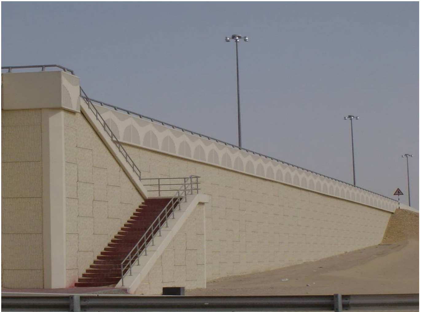
▲ The walls are up 12.0 high and designed to take a heavy goods vehicle crash barrier containment loading.
