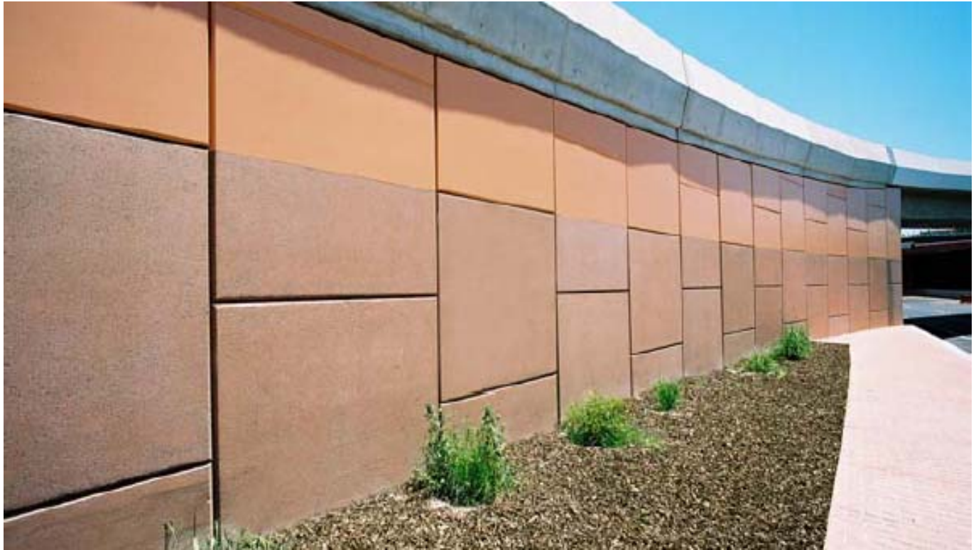
▲ Architectural Wall finish: 2 percent caramel colour with off form and sand blast finish
