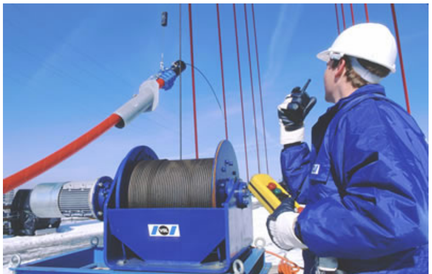
▲ The first stay pipe is erected with the first strand installed. This strand is connected at both ends to the anchorages and then stressed to raise the stay pipe. The strands are then pulled one by one through the stay pipe, connected to the anchorages and individually stressed.
