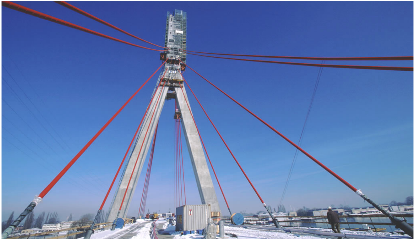
▲ No crane required : The stay pipes are moved on trolleys, then lifted from the deck to the pylon with winches supplied by VSL.
