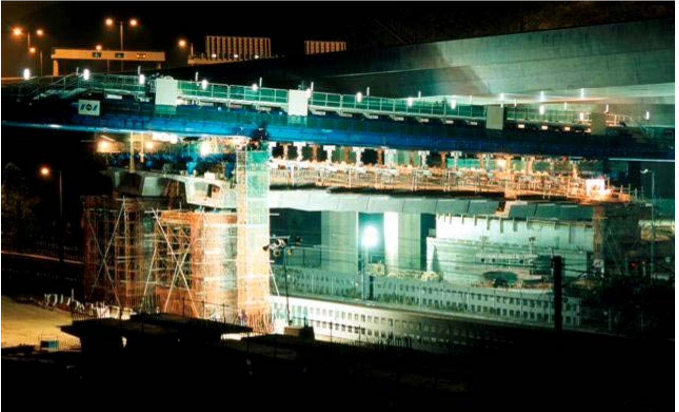
▲ Erecting precast segments for the first two spans above Hong Kong Airport Express Rail Lines by overhead girders during the nights
