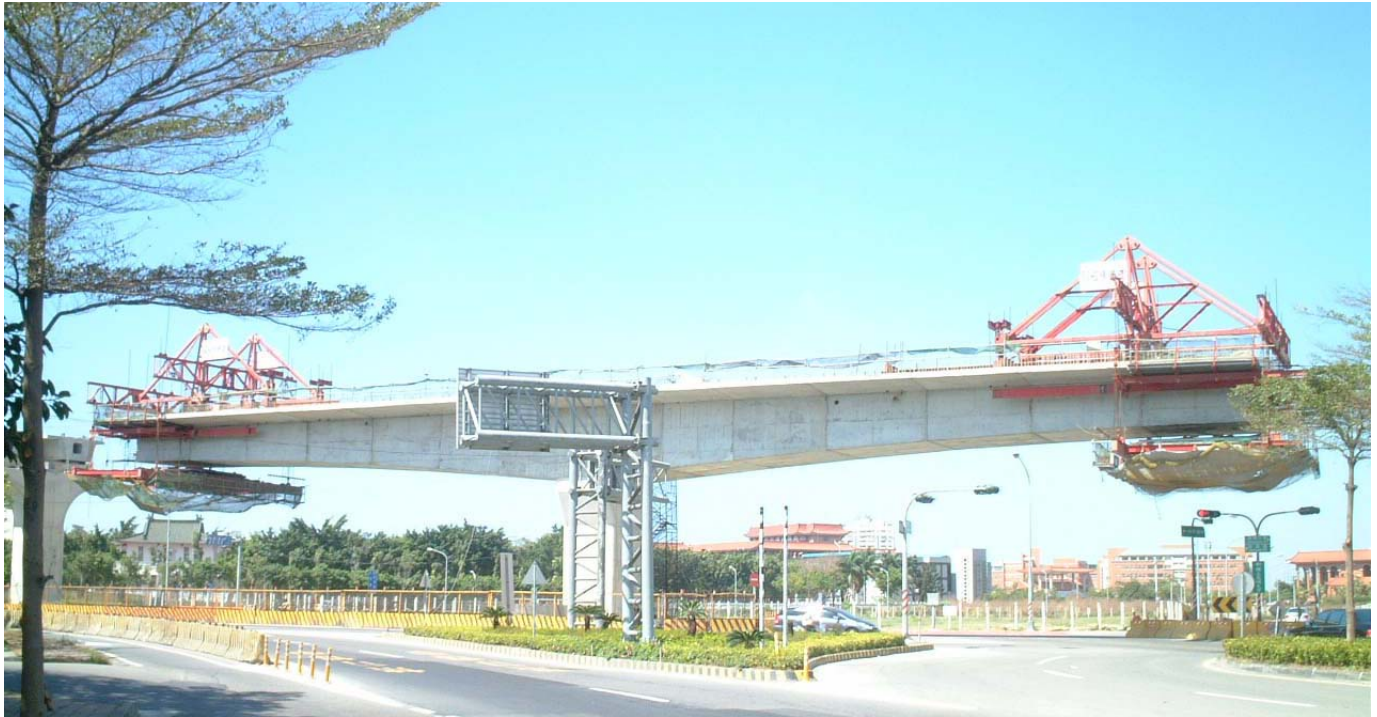
▲ VSL form traveller launched over a major road at Bridge No. LER36.
