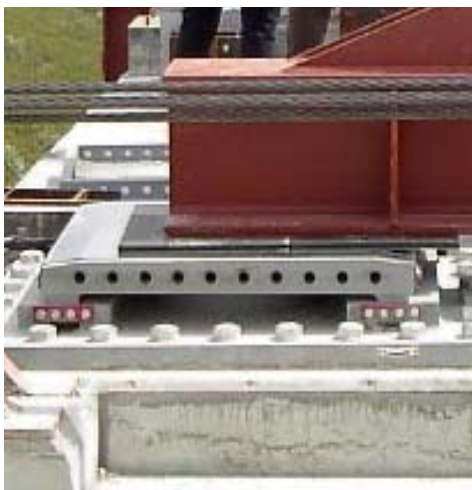
▲ A free-sliding bearing placed at the abutment
